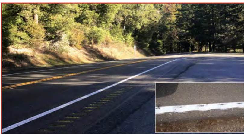
Figure 4-29. Centerline and Edge Line Rumble Strips and Rumble Stripes (Inset)
