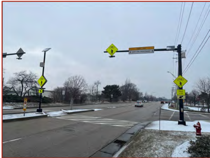
Figure 4-2. RRFB at a Multi-Use Trail Crossing
