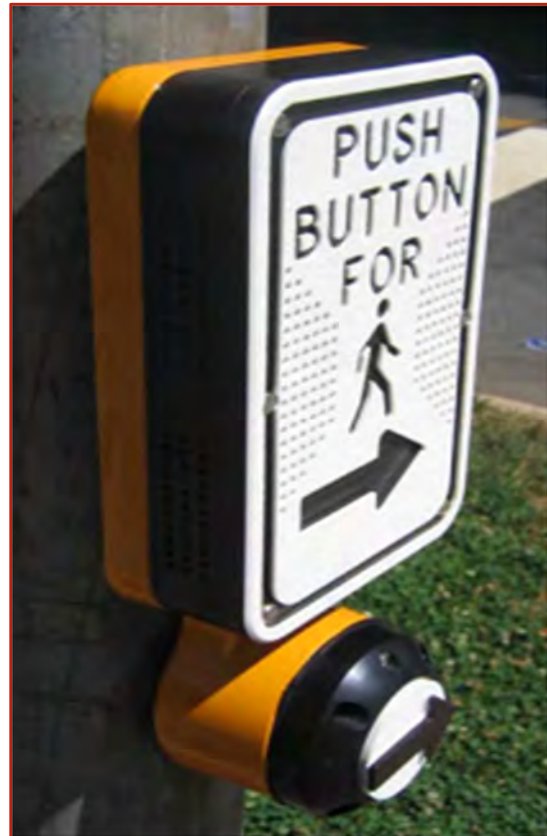
Figure 4-5. Accessible Pedestrian Signals
