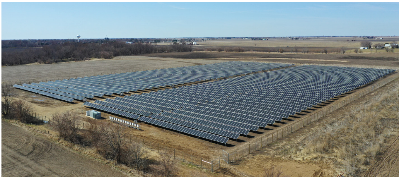
Figure 19. The 2.7MW Somonauk Road Community Solar project was developed in Somonauk by Nexamp, Inc. The project began producing clean energy to benefit subscribers in the ComEd territory in March of 2021. Image credit: Nexamp, Inc.
