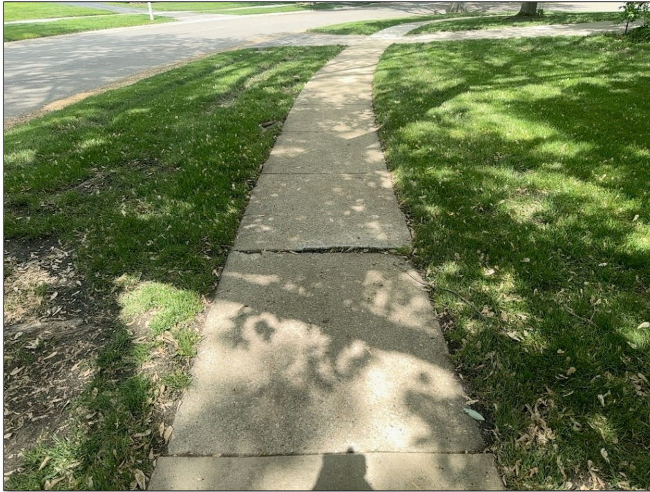
FIGURE 6. EXAMPLE OF SIDEWALK WITH TRIPPING HAZARD
