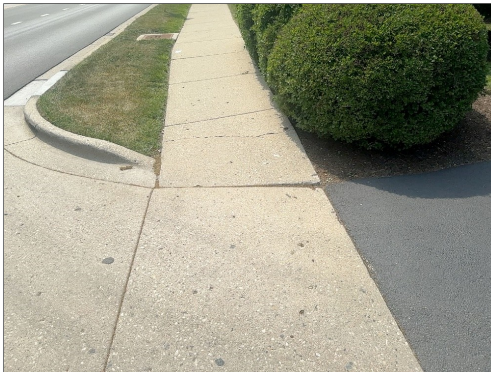
FIGURE 5. EXAMPLE OF SIDEWALK WITH SEVERE CROSS SLOPE
