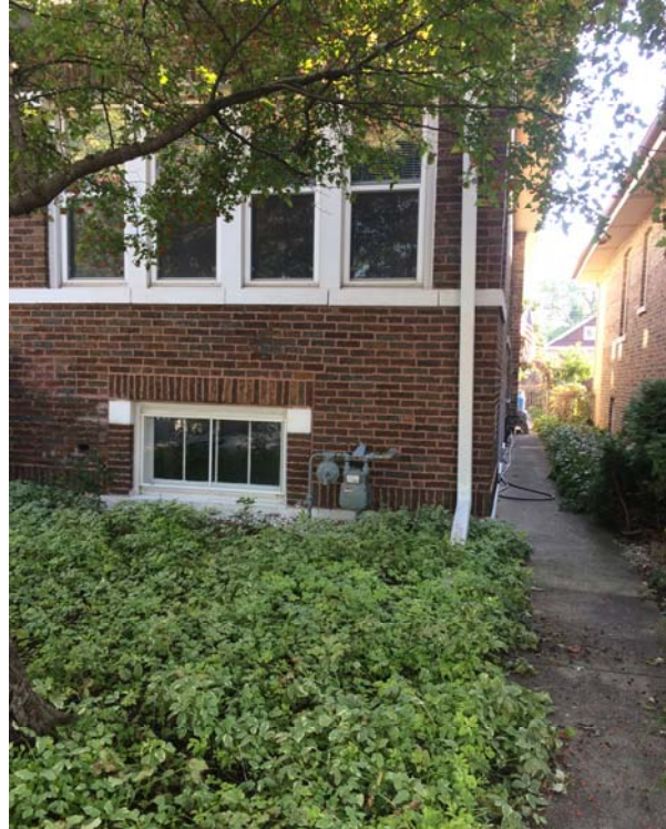
Example of downspout disconnection to a rain garden in Berwyn.
