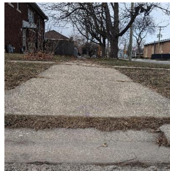
_____ Broken curb ramp (e.g. uneven walking surface)
