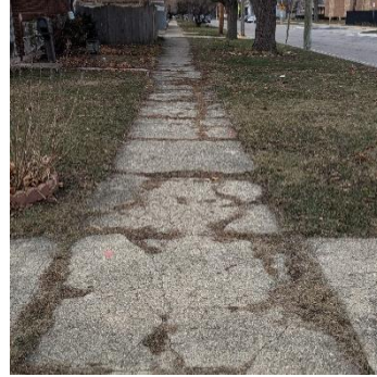
_____ Poor Surface Quality (e.g. broken sidewalks)
