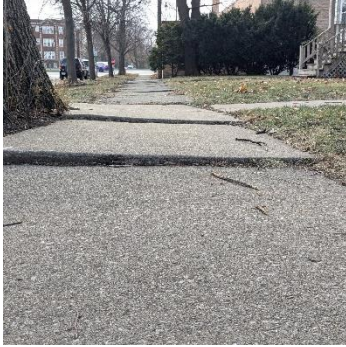
_____ Trip Hazards (e.g. uneven sidewalk panels)
