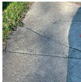
_____ Broken curb ramp (e.g. uneven walking surface)
