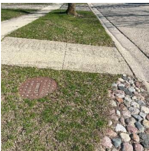
_____ Curb Ramp Grades (e.g. steep grade between the roadside sidewalk and the street)
