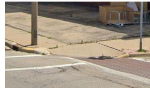
Curb Ramp example with adjacent painted cross walk. Also adjacent sidewalk obstruction.
