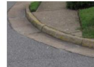
Sidewalk/Curb interface with missing ramp example. These locations were classified as a type of non-compliant curb ramp.
