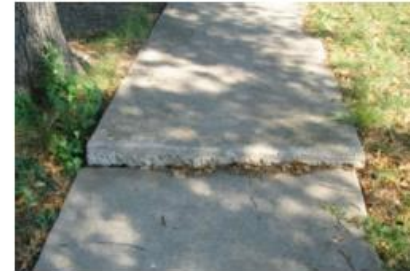
Trip Hazard Example
