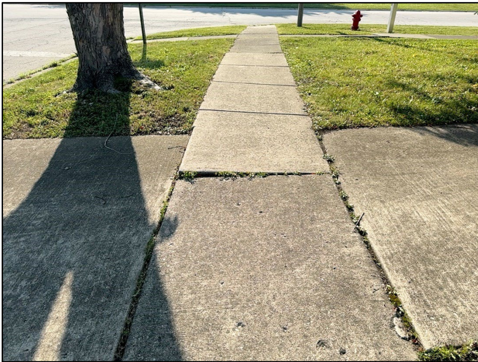
FIGURE 5. EXCESSIVE CROSS SLOPES
